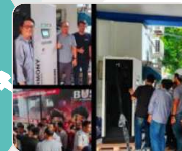
DC charger installation in Indonesia
