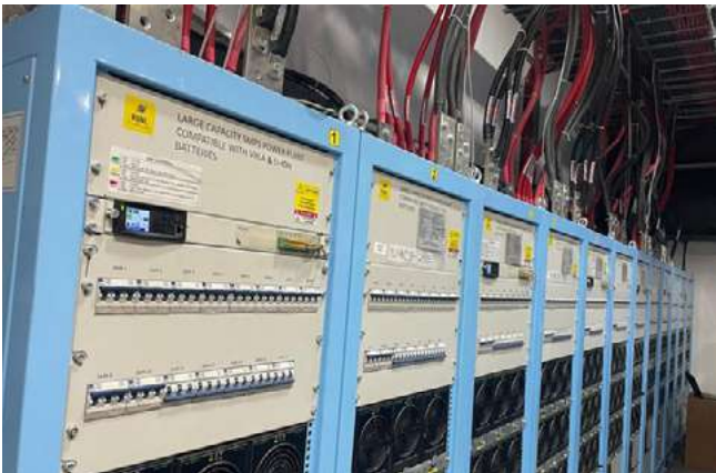
Large power solutions for powering switching centers (<50kW), cable landing stations
